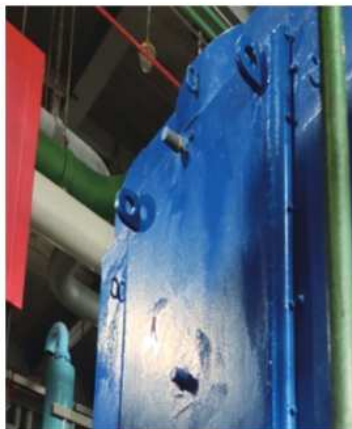
Condensate Pump Monitoring – Power Plant
